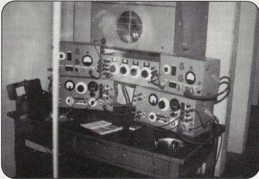
Communications room at the Churchill Bunker in London. During World War II, British Prime Minister Winston Churchill directed his country's war efforts from here—and kept in touch with U.S. President Franklin Roosevelt on a secure phone installed in his bathroom!
