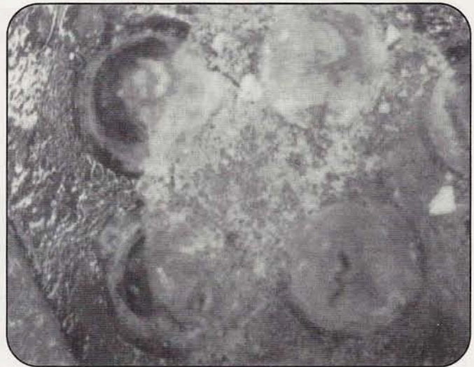
Photo D. An advanced case of corrosion caused by water condensation. The solder material has broken down into conductive metal-based salts. Under the right conditions, this can result in shorts to adjacent pins.
