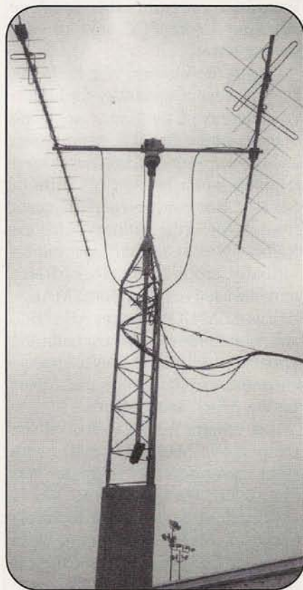
The impressive satellite antennas at W5RRR are completely computer-controlled, allowing hams at the station to concentrate on communicating with the orbiting astronauts rather than pointing antennas.
