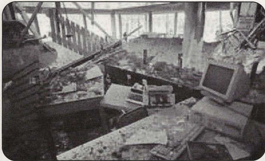
Photo A. Bomb-damaged office building somewhere in Yugoslavia. (Downloaded from a Yugoslav Web site)
