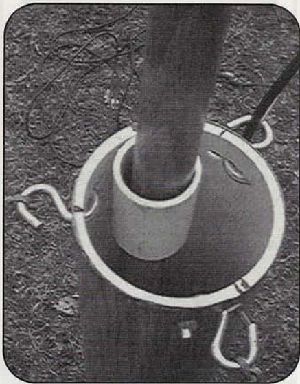
Photo C. Close-up view of the top of the 4-inch pipe section. Note the marks above the S-hooks that show where the hooks will go. The 1-inch mast pipe sits inside a 1-1/2-inch sleeve section and, 2 feet down in the pipe, a 1-1/2-inch end cap. These are both screwed into the base pipe. See text for details.
