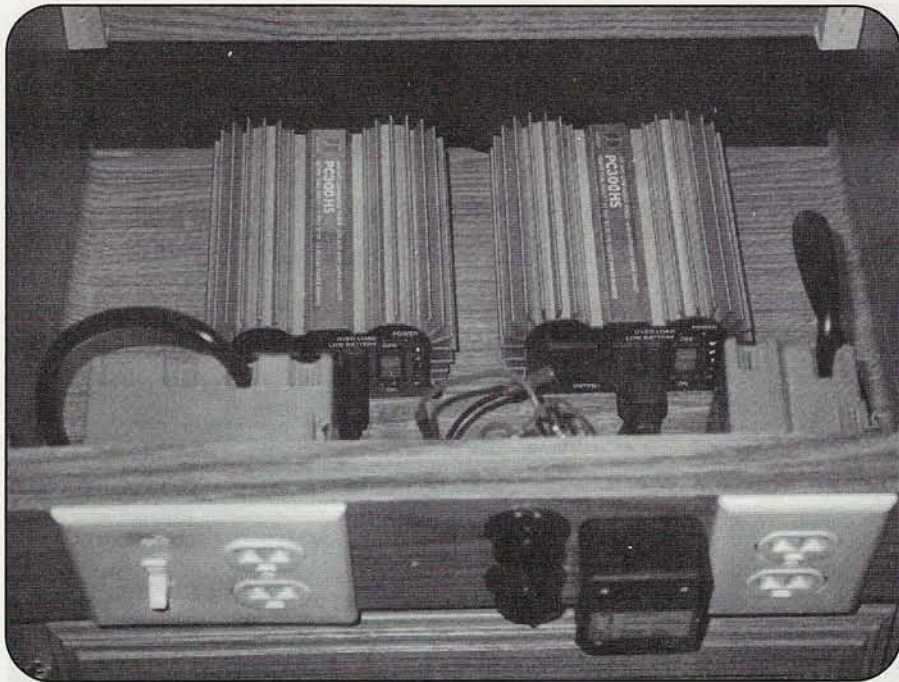
Photo D. The two 300-watt DC-to-AC inverters sit on a second added shelf. They are accessed by removing the wooden top.
