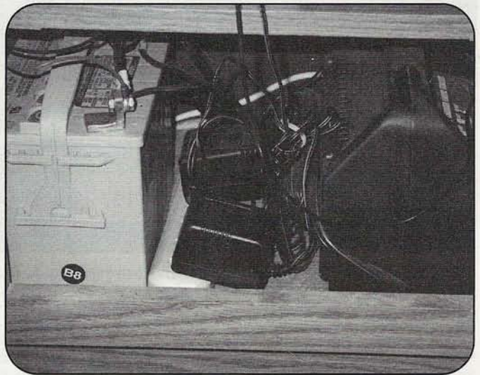
Photo C. Base of emergency power unit. Deep-cycle marine gel-cell battery is on the left, an AC power distribution strip is in the center, and the 2/110-amp charger is on the right.
