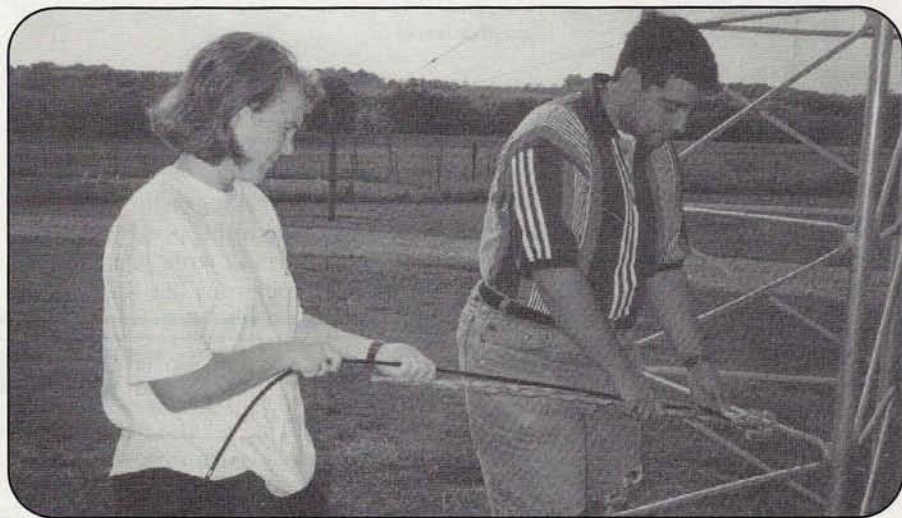
Photo A. Dori Baker, W8YR, and Saleem Banatwala, KC5UHS, begin wrapping Phillystran guy cable in "big grip" steel wrapper. (Photos courtesy of the author)
