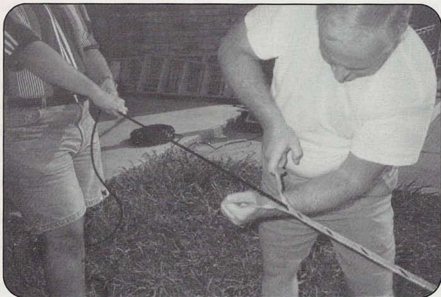
Photo E. As you approach the end of the "big grip," the cable becomes quite stiff and may be difficult to work with. The good news is that you're almost done.
