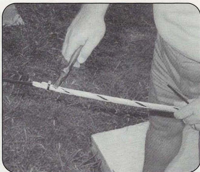
Photo G. A heavy-duty tie-wrap at the top end of the "big grip" will ensure that everything stays in place and that you don't have to repeat the wrapping process (except on the other cables!).
