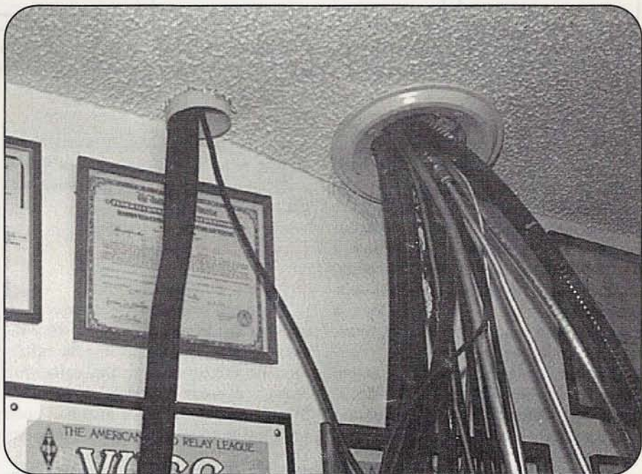
Photo A. Some, but not all, of the author's coax runs. WA5VJB currently has 31 antennas: 20 outside and 11 inside. That's a lot of cable!
