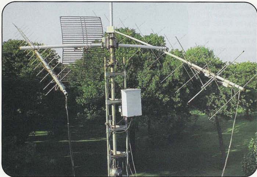
Photo 3. Cross-polarized (CP) antennas provide good, general-purpose service for satellite and terrestrial communications. Note the tips of the 2-meter antenna (left) elements are perpendicular to the elements of the 70-cm antenna. This improves isolation and minimizes desensing. (Photo courtesy WA9AFM)
