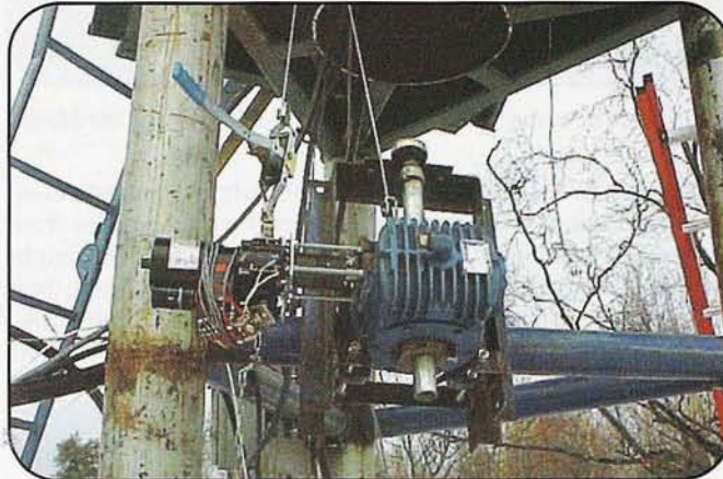
Photo 11. The surplus 5-HP right-angle gearbox for the main azimuth drive.
