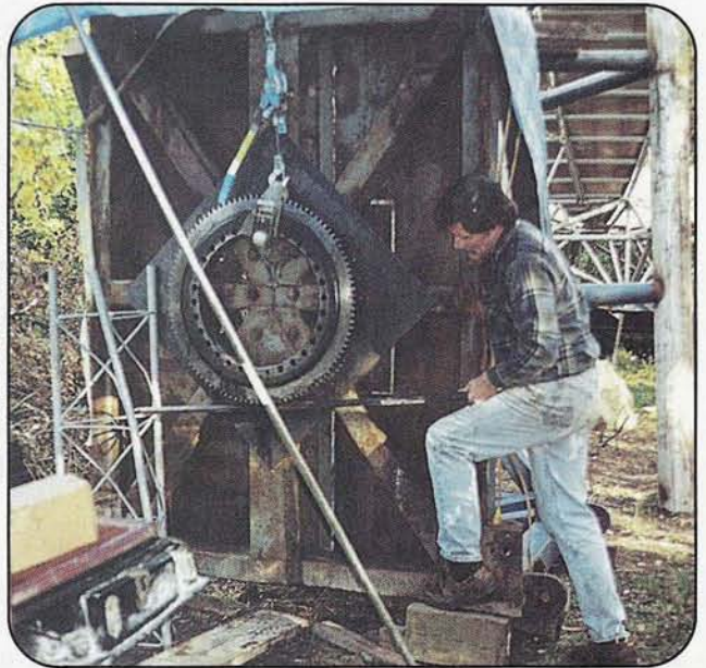
Photo 4. How one man does a two-man job—attaching the crane bearing to the elevation platform.
