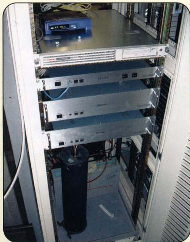
The FRRL D-STAR rack. From top to bottom are the WRT-54G running Linux; then the Linux server running the ICOM gateway software, the ICOM RP2C Controller, and the RP-2000 2-meter repeater; and at the bottom the RV-4000 442.100-MHz repeater. Also visible at the bottom of the relay rack is the 440 duplexer and bandpass cavity. (Photo courtesy of Greg Braun, N9CHA)
