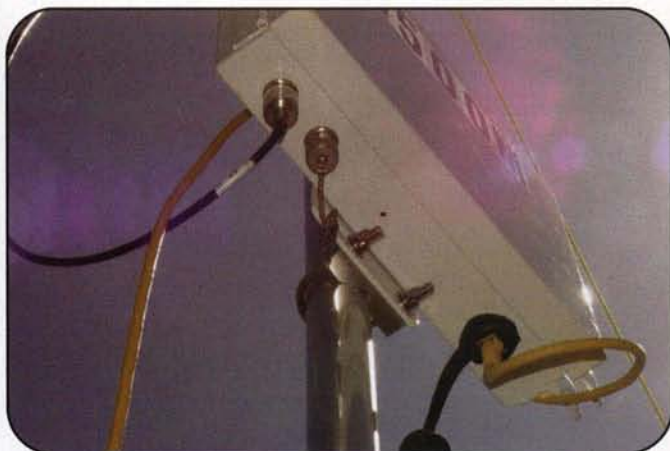
A closer look at the battery-powered WRT54G. (Photo by KD5OUG)
