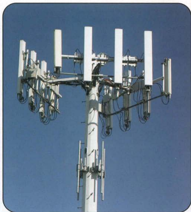
This Cingular Wireless tower has three sets of directional antennas to increase channel capacity by dividing coverage into multiple sectors. The antennas do not have sufficient directivity to provide accurate angle-of-arrival information on incoming signals. (Photo by Joe Moell, KØOV)
