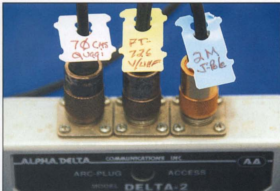
Photo 2. This photo shows how the plastic ties from bread/bagel bags can be used to tag smaller coaxial cable such as RG-8X, RG-58, and RG-59.
