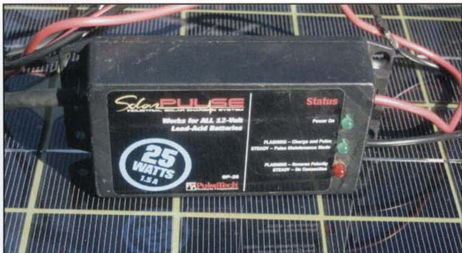
Photo 2. PulseTech SP-25 solar-panel system.
