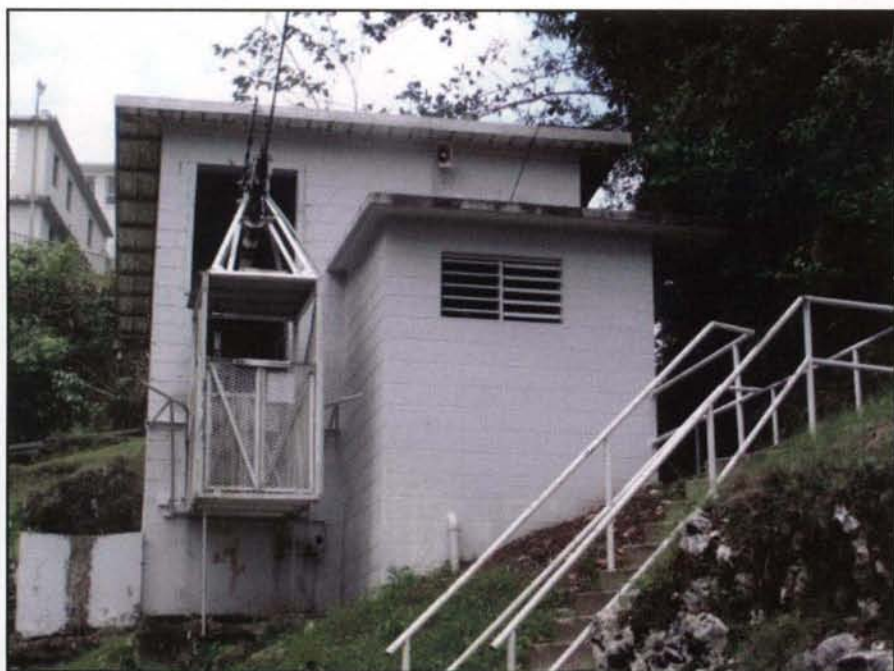
Gondola at the ground station.
