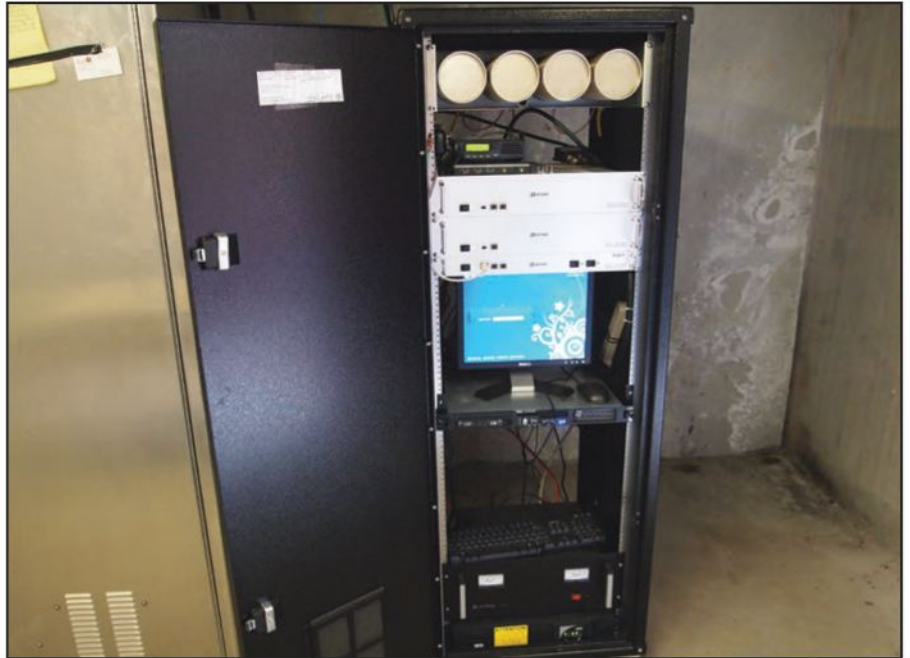
The D-STAR repeater stack at Rowan University in Gloucester County represents a typical layout.
