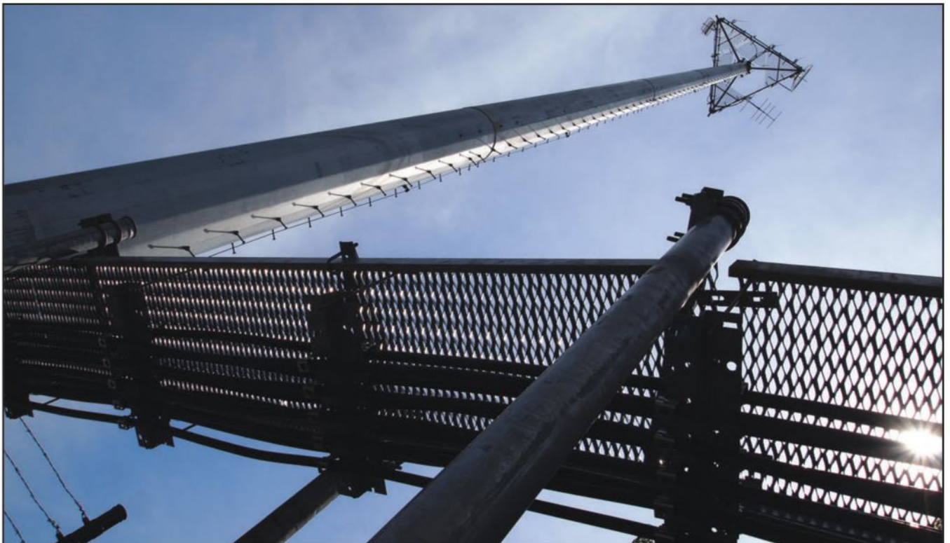
View of hardline cabling and monopole with candelabra.
