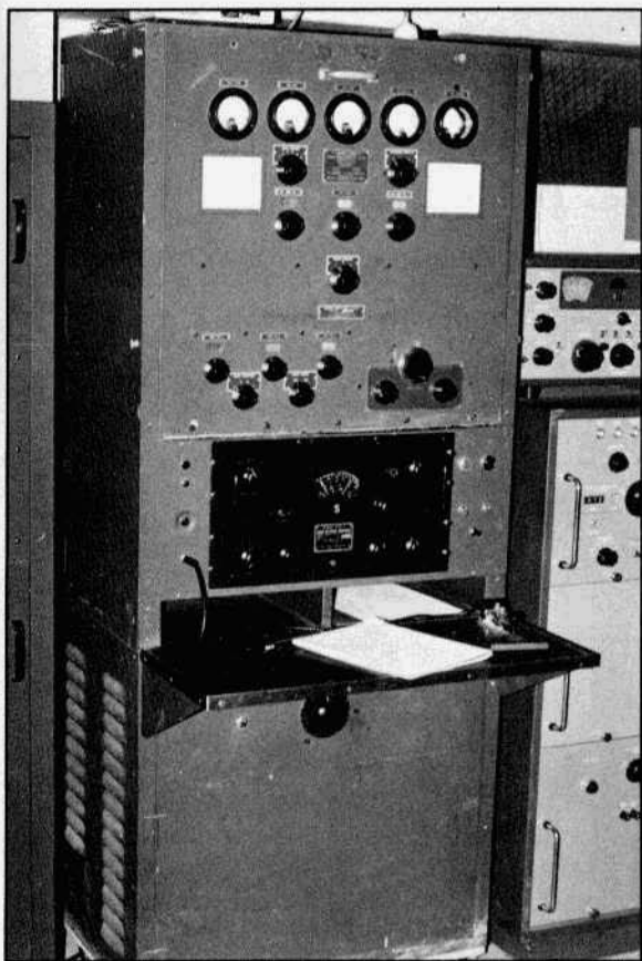
FT-102 set in KW11's shack. To the right is a GPT-750 transmitter with a GPR-90 receiver sitting on top of it.
