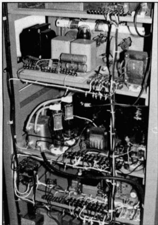
Rear view of transmitter.
