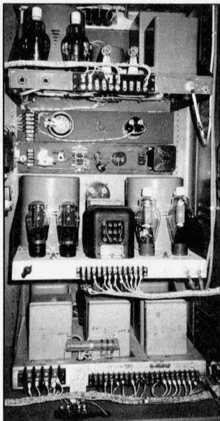
Rear view of decks below the RF deck; high-voltage power supply, filament control, modulation monitor, modulator and low voltage power supply.
