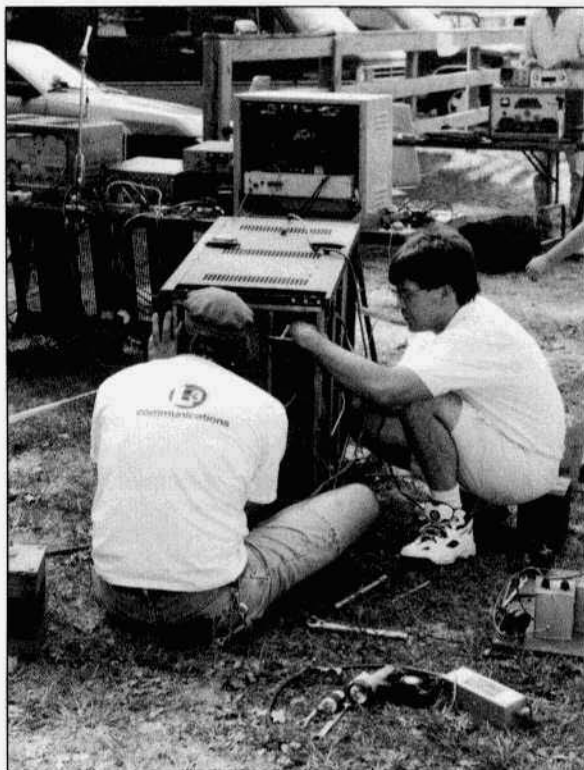
Dave, KB2APE, installs the iron and the tubes for the modified BC-610—pair of 813s driving a single 833A.
