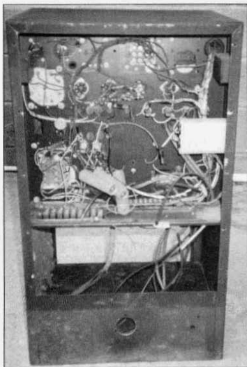
A rear view of the power supply deck— a real mess!
