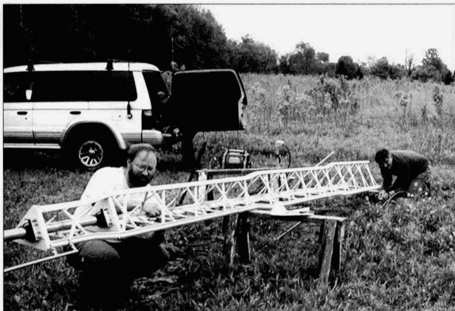
A trio works assembling the Hy-tower. The generator provides power for the soldering iron. Each aspect of assembly was delegated to one person for completion.
