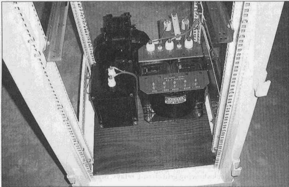
View of power supply installed in cabinet. The transformer in the upper left corner is the modulation reactor.
