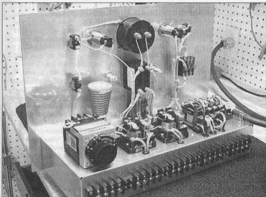
Rear of control deck showing Agastat timing relay on left, low voltage relay, step-start relay and plate relay. The cone shaped ceramic device in rear is the step-start resistor.
