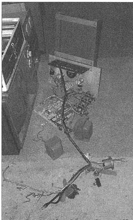
Figure 1: Here is the main wiring harness as it looked after it was removed from the rig for cleaning and inspection.
