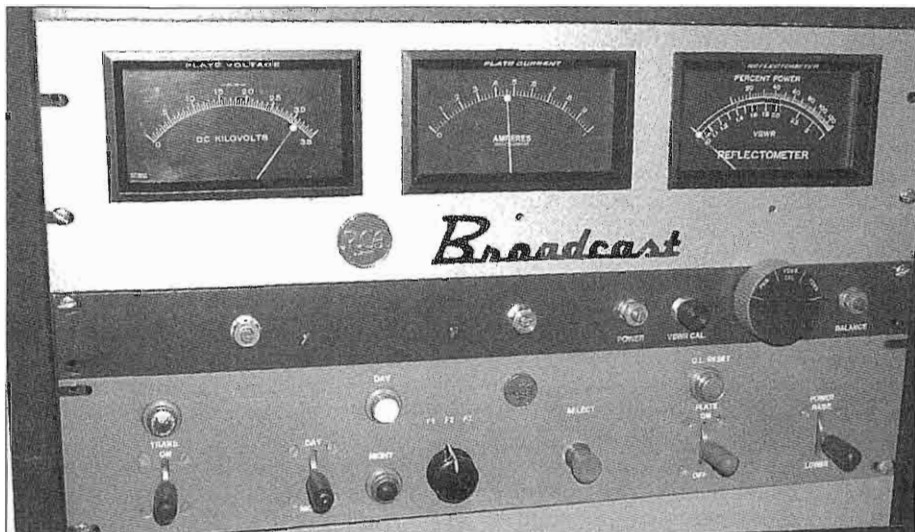
Figure 1: Front view of the completed, custom-built BTA-1R1 remote control panel that is mounted in an accessory cabinet at the AM operating position. The transmitter is operating at full power, but the VSWR meter is not yet connected.
