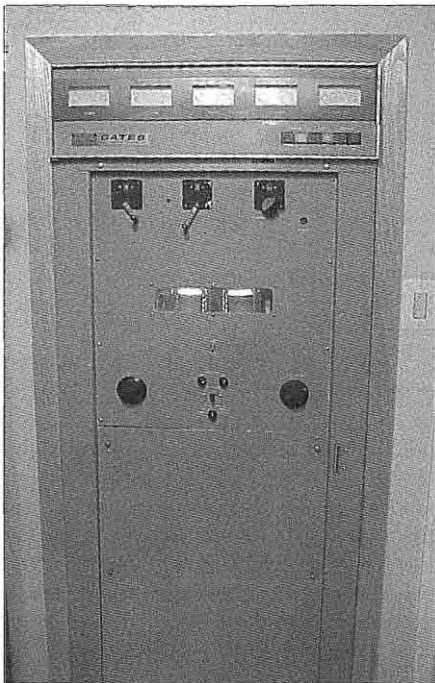
This modified Gates BC-1H has been built into a wall, as was typical with broadcast station installations.
