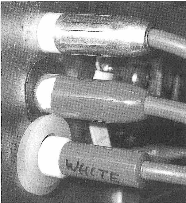
The "as found" high-voltage connectors on the rear of the RF unit.
