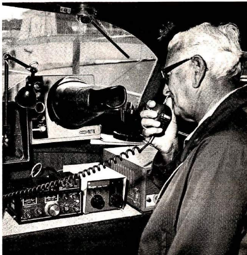
An amateur radio installation on the bridge of a power cruiser. The small white box to the right of the transceiver is an antenna tuner which permits the use of a random length of wire for all bands. The equipment is secured by brackets.
