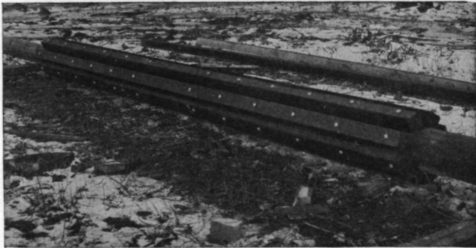
FIG. 3.111. A butt-spliced pole ready for erection. ( Photograph courtesy of RCA Communications, Inc. )
