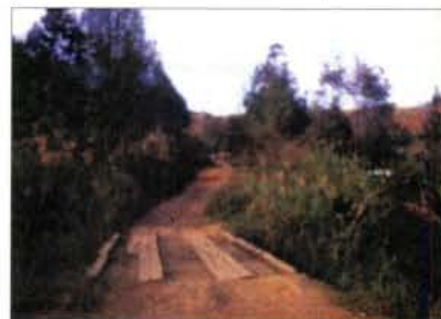
Fig. 2: Example of one of the more rickety bridges which "frightened the living daylight" out of Tony!
