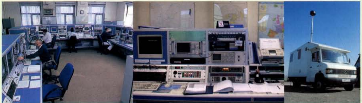
● Fig. 4: View of the main control room during a day shift. The Baldock station operates 24 hours a day, seven days a week throughout the year. It played a very important part during the 11 September terrorist attacks on the New York World Trade Centre's twin tower by Muslims in 2001, when the Transatlantic Aeronautical h.f. services were disrupted by interference (see text). (photo courtesy of the RA)
