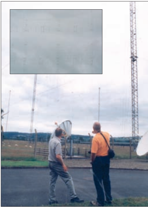
● Fig. 3: Dwarfed by the main masts at Wooferton, Dave Porter G4OYX describes to Kevin G7TZC how the multiple wire dipole, stacked array antennas work together with their associated curtain reflectors. (see inset and text). The satellite dish antennas are used for transmission and reception of programmes to be re-broadcast, onward broadcasting abroad, and linking to other former BBC transmitters around the world (see text). 'Ground Maintenance Staff' (sheep) can be seen at work...keeping the grass short amongst the antennas.
