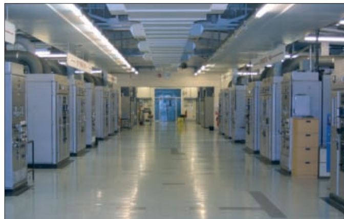
● Fig. 7: The main transmitter hall at Wooferton. Unusually, because of the high water table...the transmitters do not extend below floor level (see text). Photo by Kevin Nice G7TZC.
