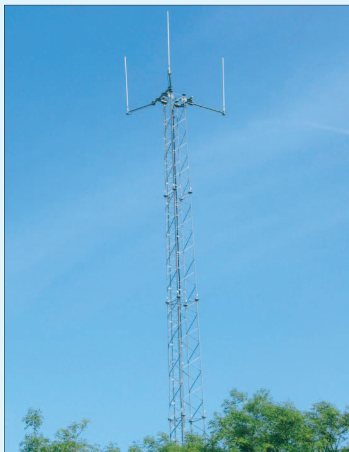
● The gain of the proposed antenna system of this TETRA mast, seen here under construction about 1km from Gordon's home in Brixham, will be 8.5dBd, putting the capture area around half a square metre at a wavelength of 0.75m.
