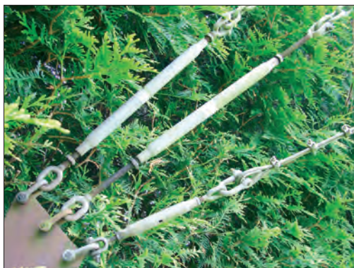
● Fig. 2: Three support wire ropes each with their own adjusting turnbuckles, are attached to a substantial steel plate (via D-shackles). A single large concrete ground-anchor provided security for ropes.
