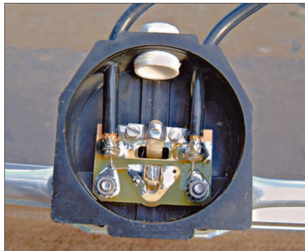
Fig. 3: Inside the feed-point box, showing the two ends of the pre-assembled matching section of coaxial cable.
