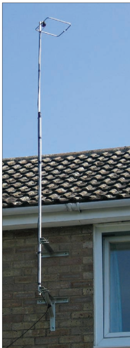
Halo on the pole fixed with pvc tape!
