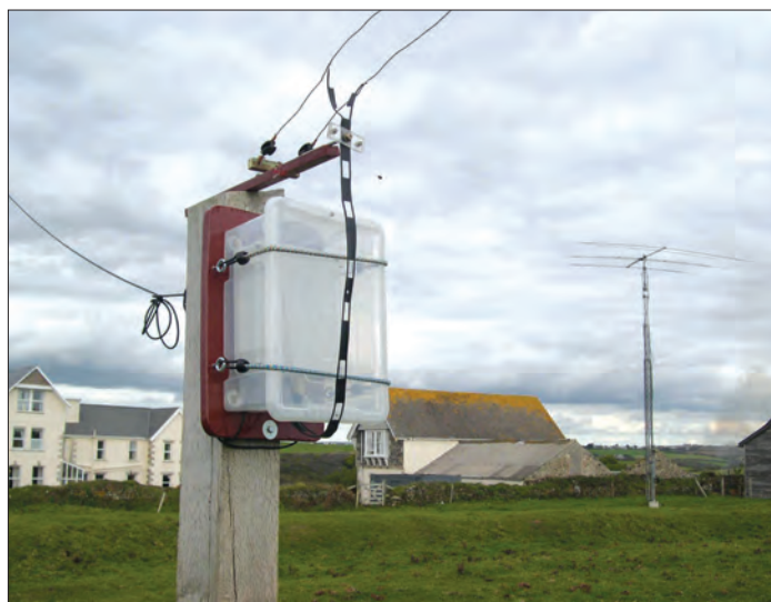
Fig. 4: The SGC-239 mounted - and fully weather-proofed against the Cornish weather - at the antenna-feed point.
