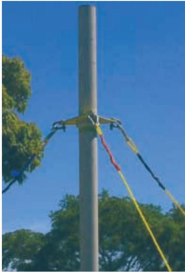
Fig. 4: The fully assembled fibreglass pole mast ready for mounting of the antenna. The ubiquitous gum trees in the background provide the much-needed shade from the glaring sun in Australia.
