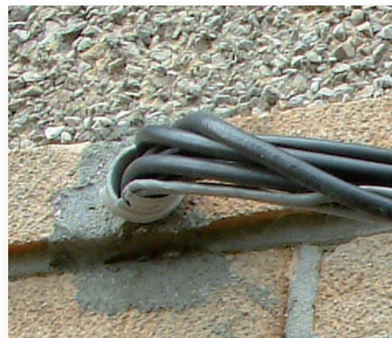
Fig. 6: Using a flexi-hose to route a number of cables through a wall.
