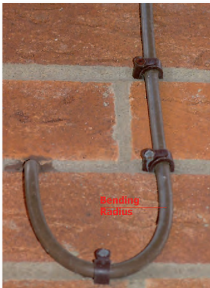
Fig. 5: Forming a 'drip loop' with coaxial cable feed stops any water from tracking along the outside of a cable.
