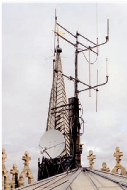
Fig. 6: Repeater antennas on the top of Lincoln Cathedral.
