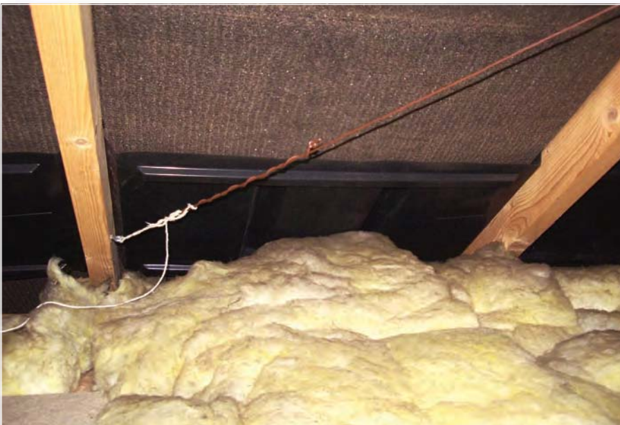
Fig. 8: Looking at the open end held tight with string attached to a roof joist.
