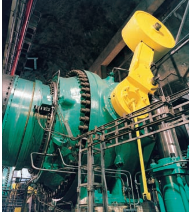
Fig. 2: The 15 ton balance weights on the valves that control the entry of water into the turbines deep inside 'Electric Mountain'.
