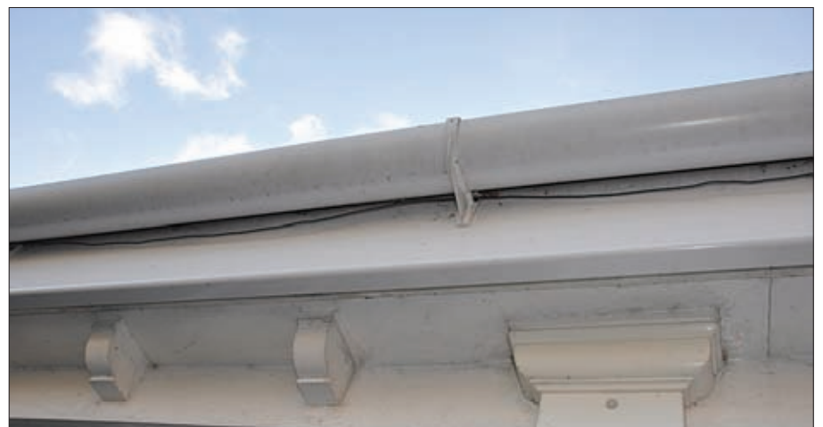
Fig. 5: A gutter mounted antenna. Changing the wire from black to white would make the antenna less visible, as would applying a little tension to prevent sagging.
