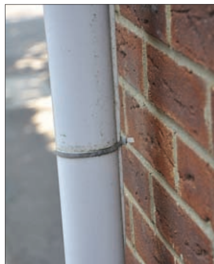
Fig. 6b: Using white feeder has helped hide the feeder still more – an even better idea would be to use matching cable ties!
