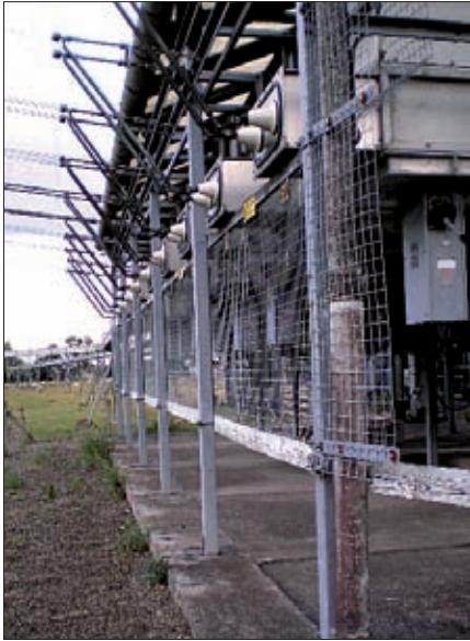
Fig. 2: A screening grid over the r.f. matrix switch station.
