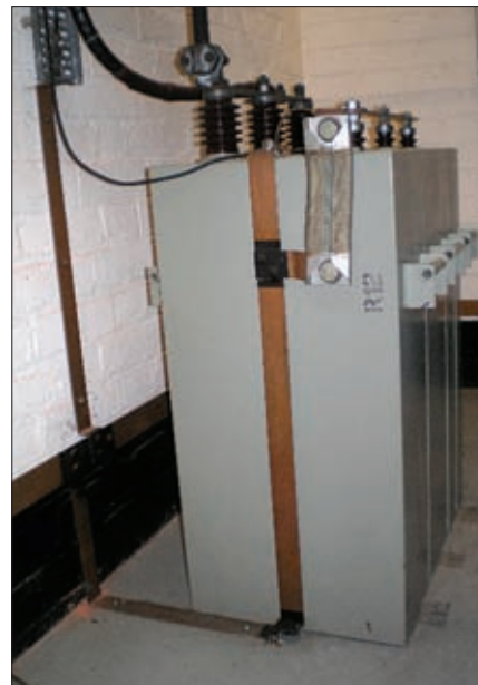
Earthing straps should be heavyweight to be effective, as shown in this transmitter cabinet at a commercial sender station.
