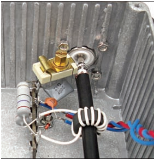
With the exception of the sensing transformer and trimmer capacitor, the components are all mounted on the 4-way tag-strip.
