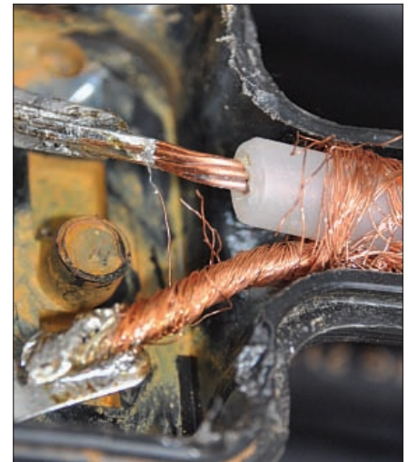
Fig. 3: Close-up photograph of the box where the feeder connects to the antenna. Note the stray wire from the shield that appears to be almost touching the centre conductor.
