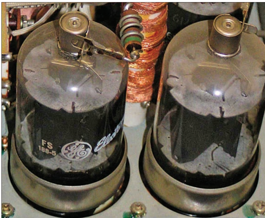
It might seem to be easy to just change the p.a. valves, but it's prudent to carry out a few voltage checks at the same time.
