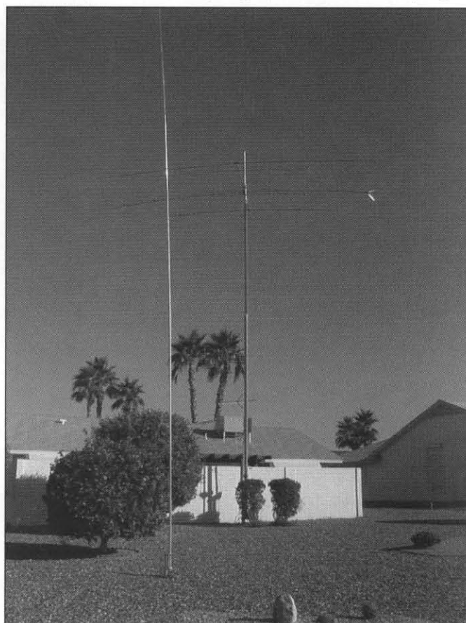
The antenna "farm" at NQ7X.
