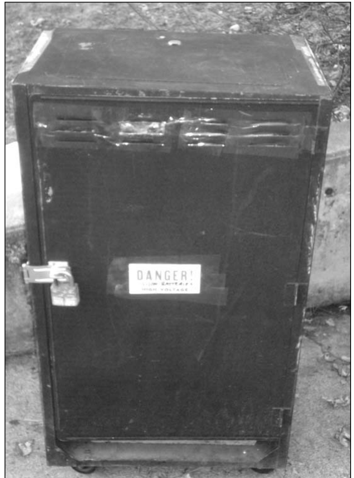
The battery safe closed and locked. And kept outdoors.
