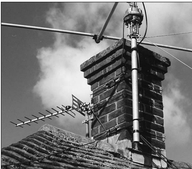
Fig 13.36: Example of a chimney lashing used to support a double-D antenna
