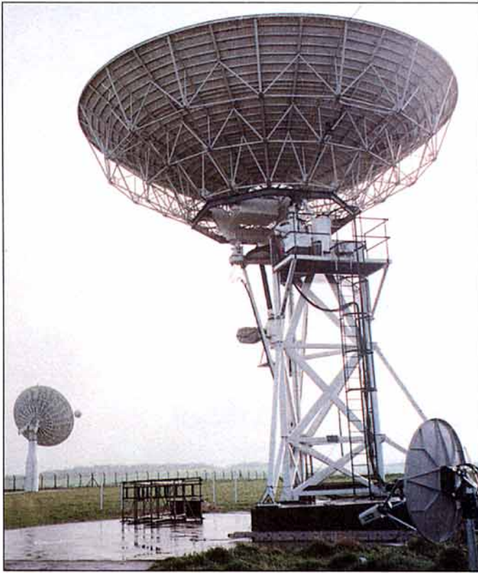
Two large dishes (12m and 10m) cover the satellite broadcast and communications bands. The one at the rear rotates at 3° per second.
