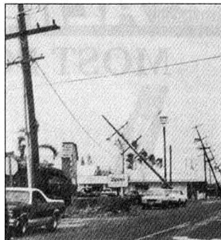
Telephone and power lines failed as hurricane Iniki struck Hawaii.
