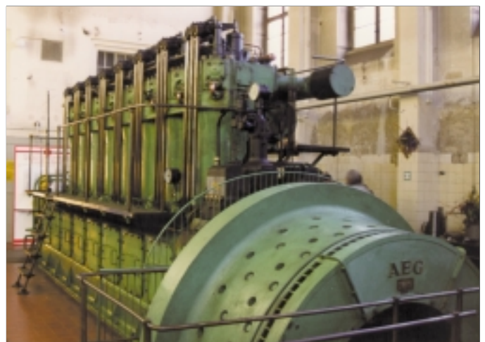
1000 PS diesel generator.
