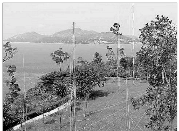
The LF antenna farm for XZ0A with the 80m 4-square and the 180ft 160m vertical far right
