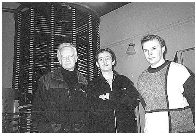
SM6BBM, SM6LKM and SM6PXJ on site at Karlsborg, with one of the large loading coils in the background.
